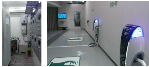
Micro-grid and Electric Vehicle Demonstration Site
