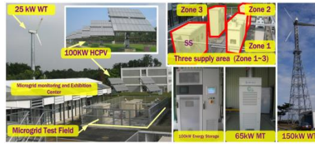
100 kW Autonomous Micro-grid Demonstration System
